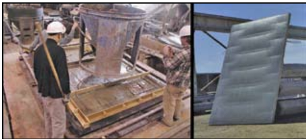
Figure 2: Full-scale formwork and completed concrete panel. Reinforcement, added to the panel, only served to hold it together and was not designed for any particular loading condition. Courtesy of C.A.S.T.
