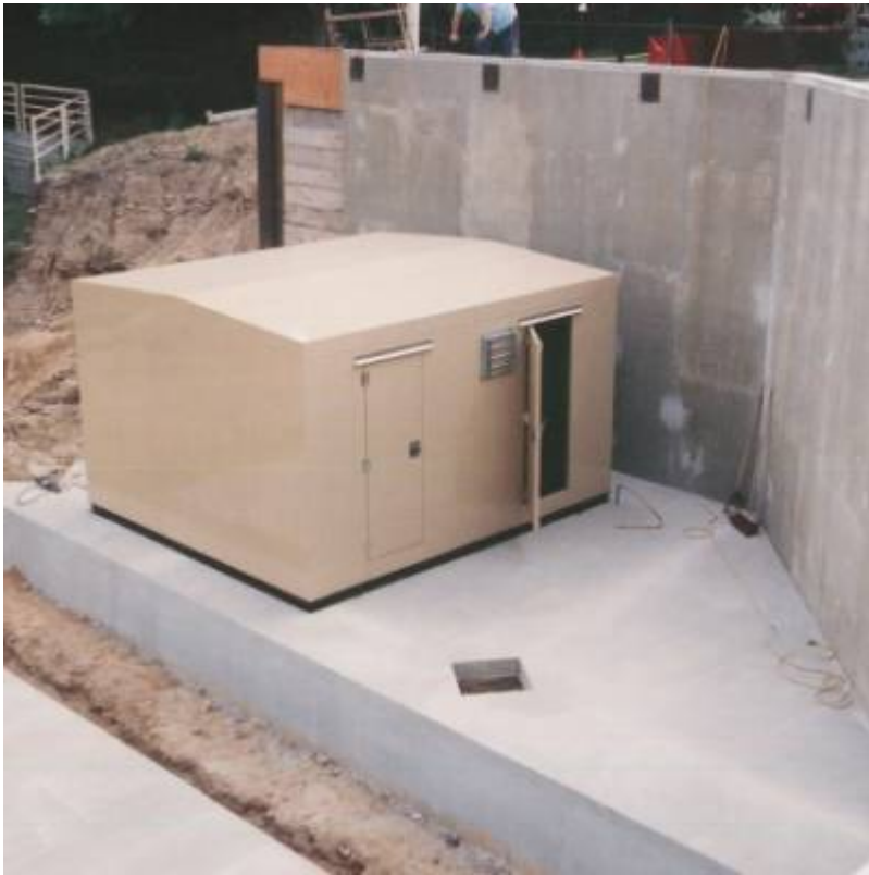
Fig. 6. Generator equipment room.
