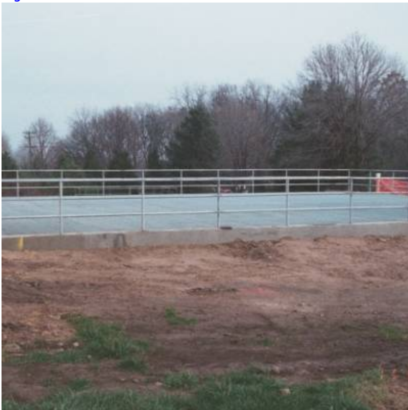
Fig. 9. Grated roof over generator installation.
