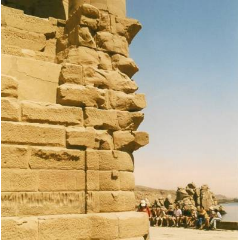
Fig. 13. Unfinished wall corner Kiosk of Trajan.
