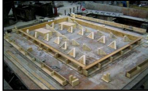
Fig. 8. Placing blockouts and interior supports prior to stretching in fabric in full-scale wall panel formwork (C.A.S.T. photo).
