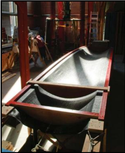
Fig. 23. Fabric mold stretched lengthwise in frame to form double-curvature funicular thin-shell vault (C.A.S.T. photo).
