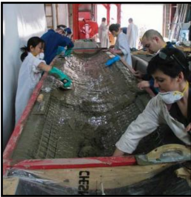
Fig. 24. Placing concrete and carbon grid in fabric mold to form double-curvature funicular thin-shell vault (C.A.S.T. photo).
